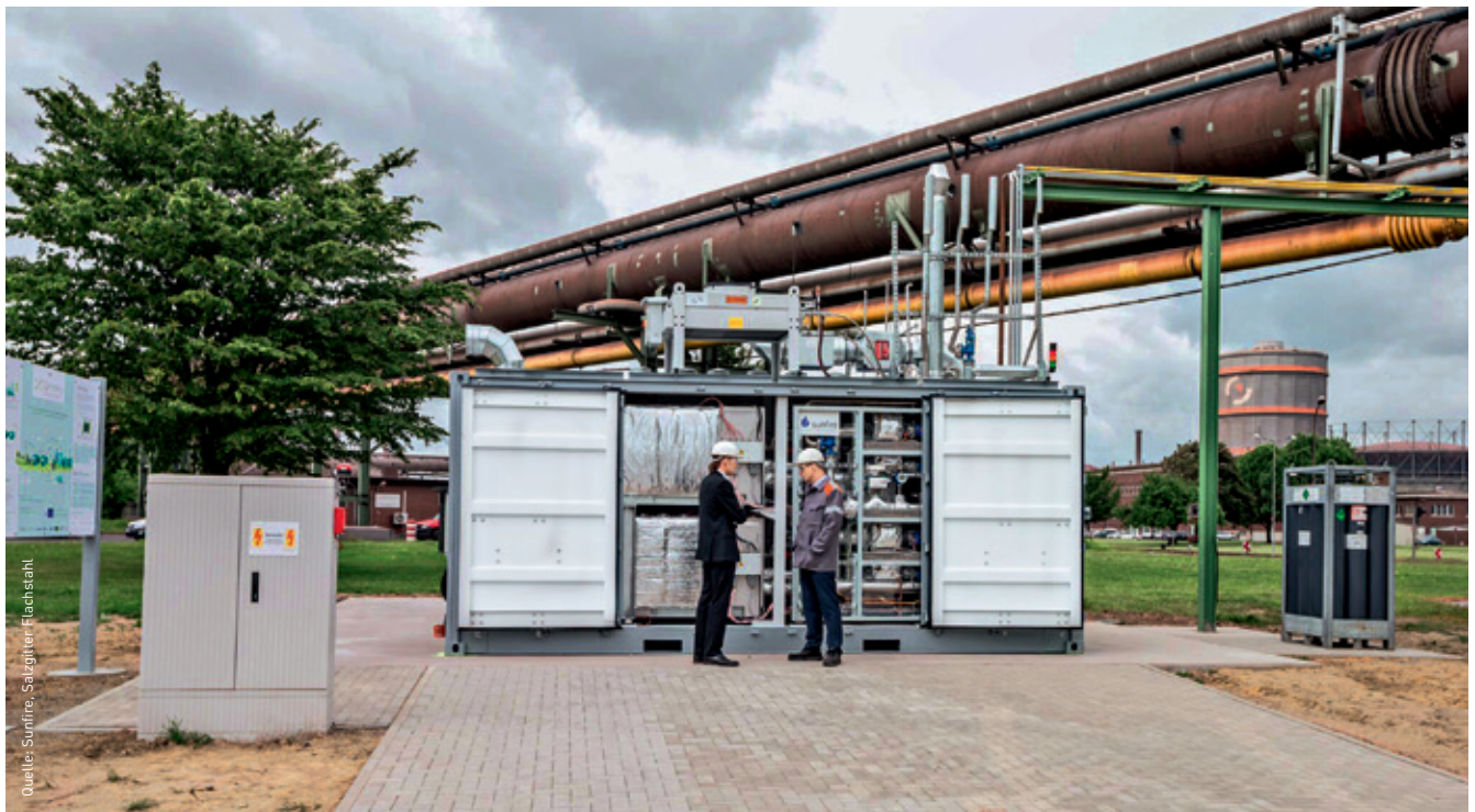
Sunfire Electrolysis Module GrInHy 1
