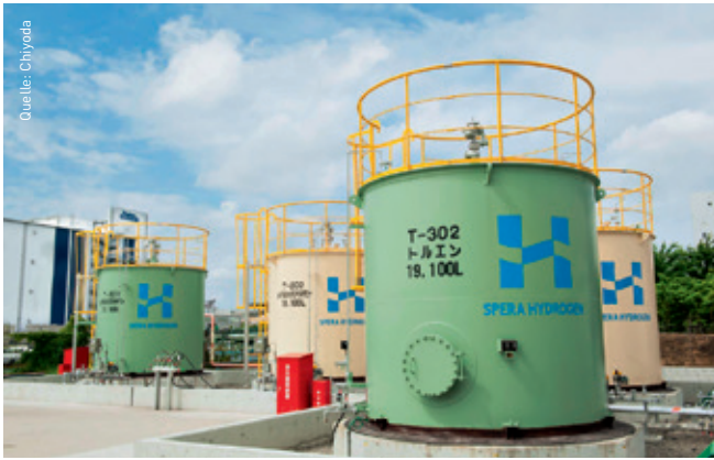
Abb. 4: Demonstrationsanlage in Yokohama
